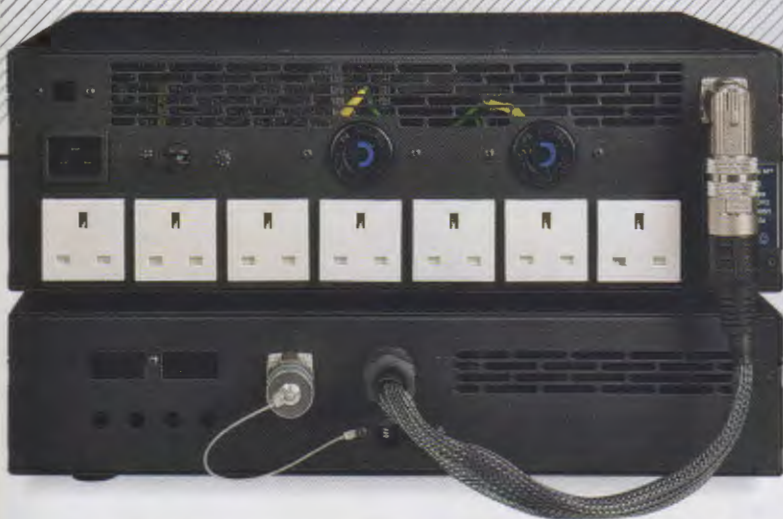
ABOVE: Seven 13A output sockets, plus two Hubbell L6-15 locking receptacles, may be used interchangeably to power source components or amplifiers. The battery PowerPack unit [below] connects via an umbilical and cells are good for 5-7 years
